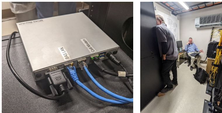
Figure 1. A Cache Poller installed at MCAS Beaufort collects operational data directly from the building automation system endpoints and sends it to the cloud for analysis.
